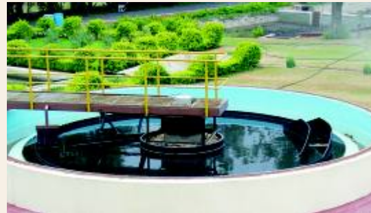
Treating waste water for reuse
