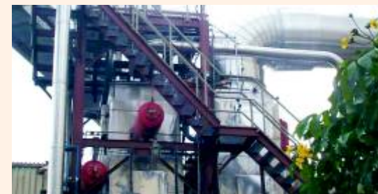
Using waste heat for steam generation
